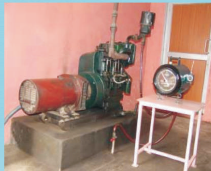
Biogas generator – Dual fuel operation with ignition by pilot fuel injection
